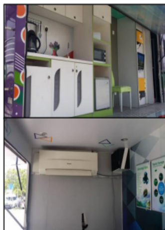
Image C5 Some electrical appliances installed in the lorry for demonstration.
