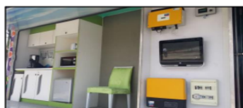
Image C4 Inverter (yellow, rectangular box shown in figure; bottom corner, right) converts the direct current (DC) into alternating current (AC).
